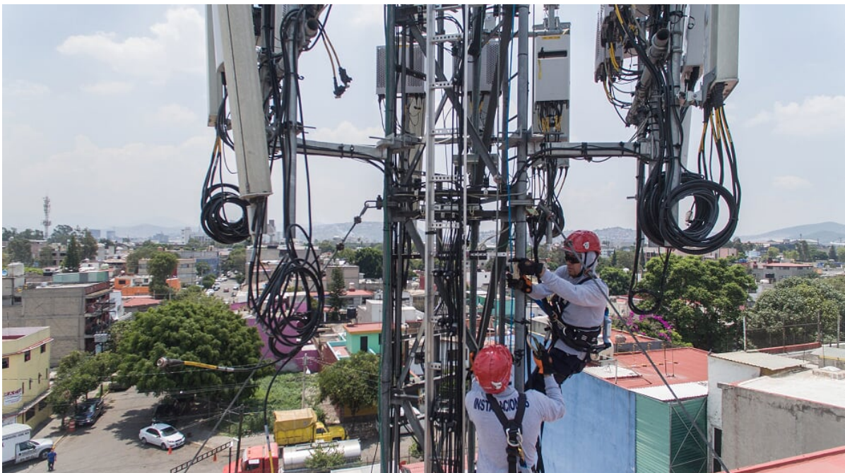
Two Panalpina technicians install telecoms equipment for a mobile network antenna in Mexico. (Photo from Panalpina)
